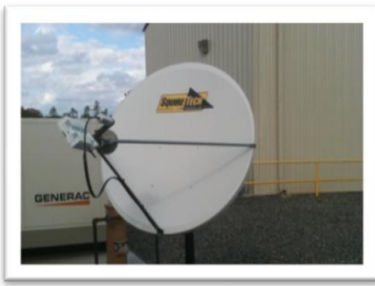
BC Antenna (backup operation)
